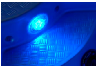
EverLite LED Lighting
