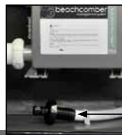
Drain / Fill Valve
